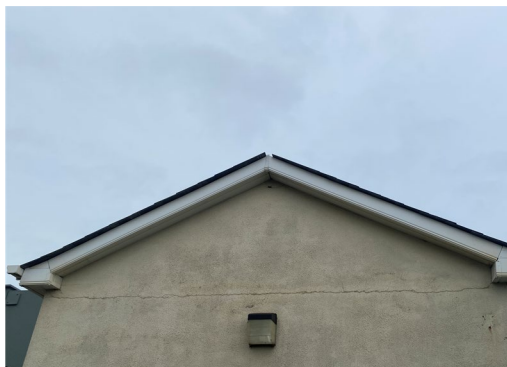
Plate 7: Crack at Top of Substation Gable End
