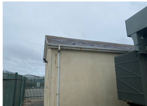
Plate 6: Missing Tiles on Substation Roof
