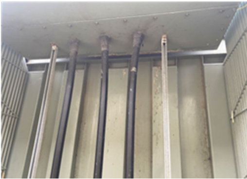
Plate 11: Bird Droppings Within Transformer
