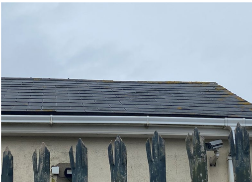
Plate 5: Lifted Tiles on Substation Roof
